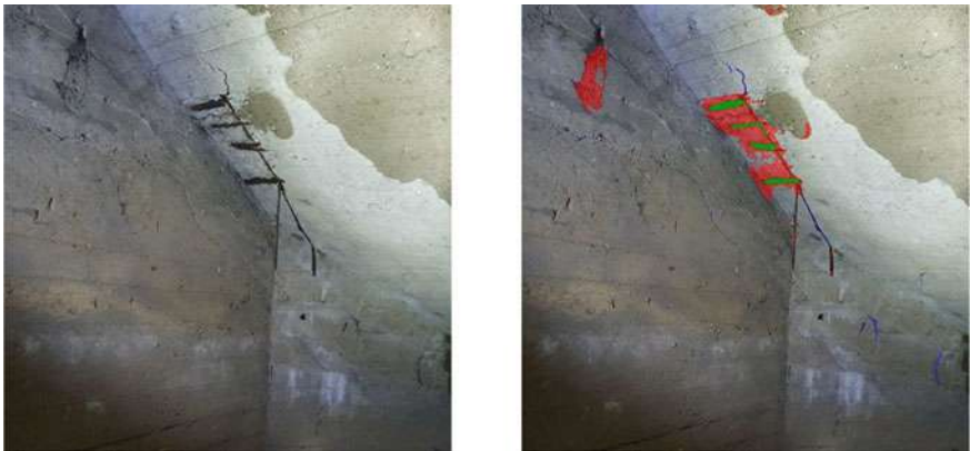
Fig. 8 Segmentation results with the FPN-Effb0 model. Red color masks are spalling predictions, blue color masks are crack predictions, and green color masks are corrosion predictions.
