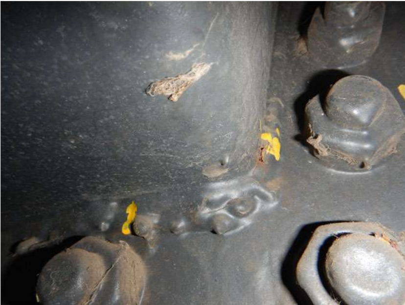
Fig. 1 Example of a steel bridge structure image where common crack detection algorithms tend to have a high false call rate.
