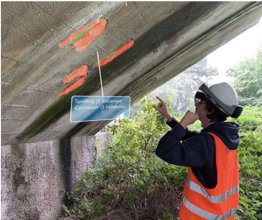
Fig. 1 Damage segmentation with the help of the HoloLens 2 on a bridge inspection mission.
